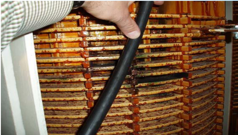
Close up of Flash Burn Marks – Coil to Coil
