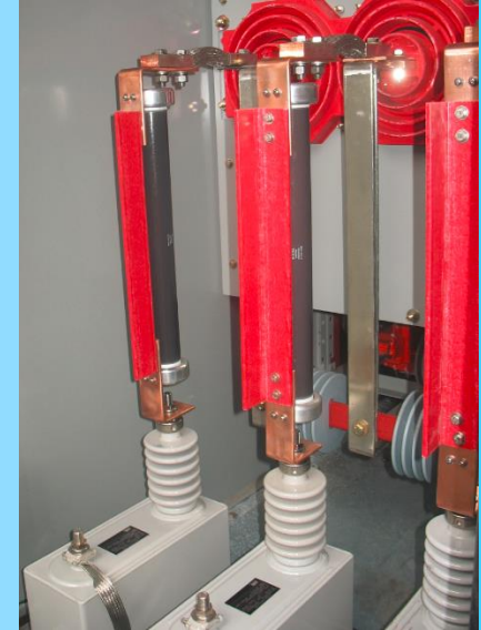
Assembly in Transformer
